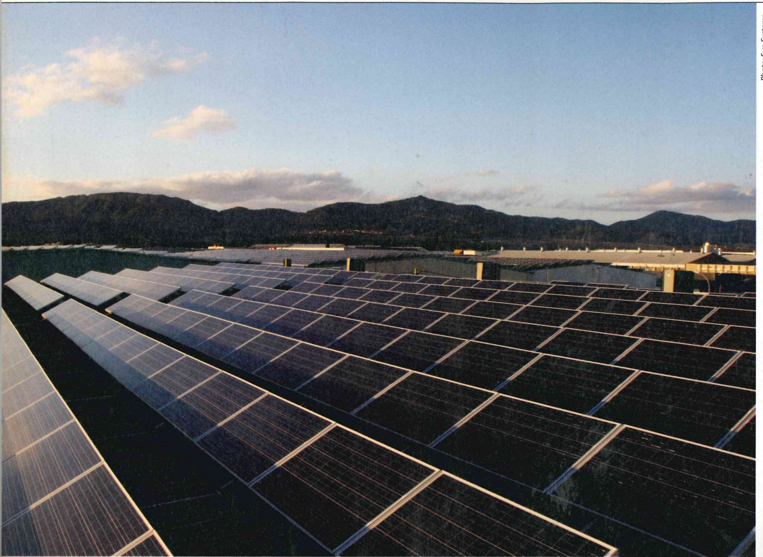
"Industrial companies are very interested in making their roofs available [for photovoltaic systems]," says Jordi Vidal, CEO of Sun Systems. Pictured above: Sun System's 1.4-megawatt-peak plant Valls in Tarragona.
